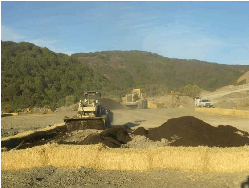
Top: Test Plot Construction at Yeager Yard Site: Applying Compost Bottom: Test Plot Construction at Yeager Yard Site: Blending Soil Materials
